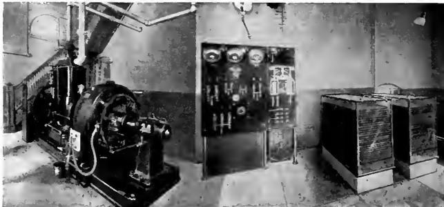
STORAGE BATTERY INSTALLATION, BINGHAMTON, N. Y.
